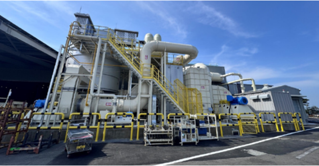
Smart Factory high-capacity RTO (Regenerative Thermal Oxidizer) facility
